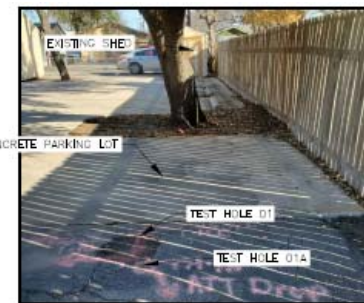
PHOTO #1 EXISTING CONCRETE DRIVEWAY AND SHE
