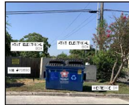
PHOTO #1 AT&T ELECTRICAL BOXES NEAR MH #70890. CONTRACTOR TO BE AWARE OF ELECTRICAL UTILITIES AND SERVICES IN THIS AREA.
